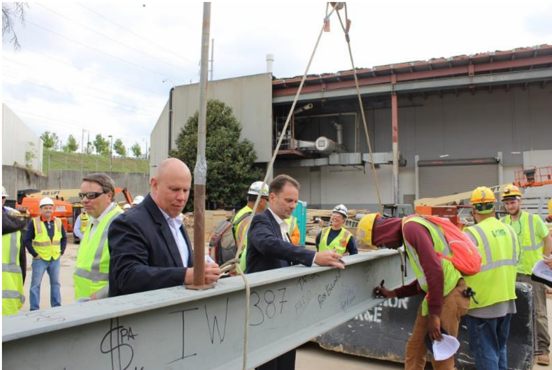
Pictured above: Project architect Gregory Mullin of PGAL (left) and Jeff Oden, GWCCA Director of Project and Program Management, sign the ceremonial steel girder before it was lifted and bolted into place.
